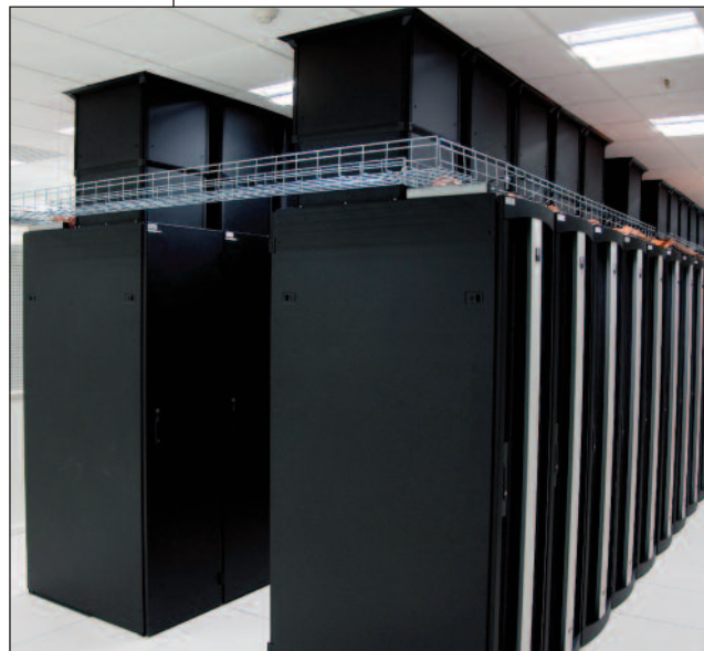
CPI's F-Series TeraFrame® Cabinet System was selected for the 5,000 square metre data centre.
