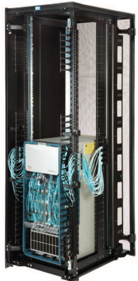
Side view of cabinet with Cisco switch
