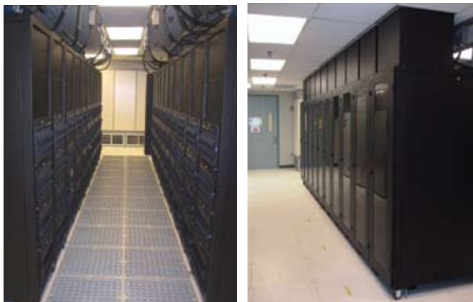
Figure 6 (hot) and 7 (cold). The basic cabinet can dissipate even more heat under appropriate circumstances.
