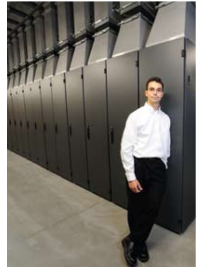
Eric Patterson, data center manager for CDW, stands in front of one of the 103 F-Series TeraFrame Cabinets that are installed in Phase 1 of CDW's Madison, WI-area facility.
