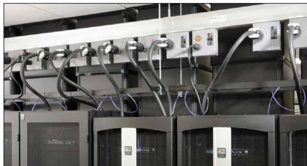
StarLine Overhead Electrical Distribution
