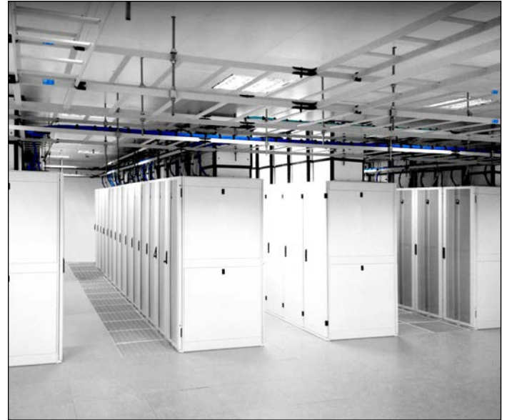
CPI's GlobalFrame and N-Series Cabinets in Glacier White brighten Oman Data Park's new, robust data center.
