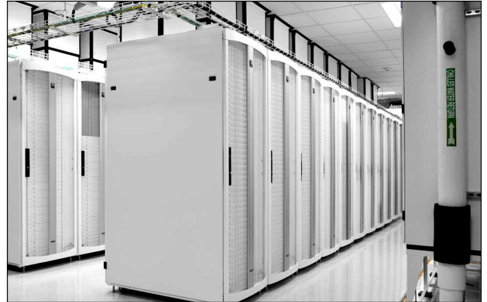
CPI's F-Series TeraFrame Gen 2 and N-Series Network Cabinets in Glacier White brighten UF Health Shands' data center and provide better visibility, while reducing power costs.
