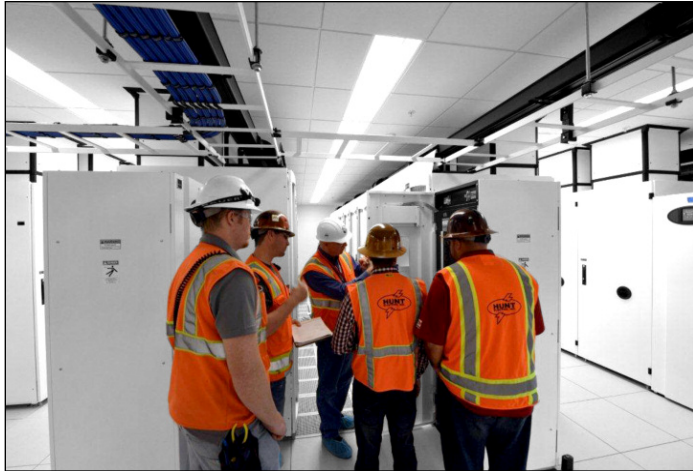
Hunt Electric's I.T.S./Data Communications Team works to layout CPI cabinets in Nu Skin's data center.
