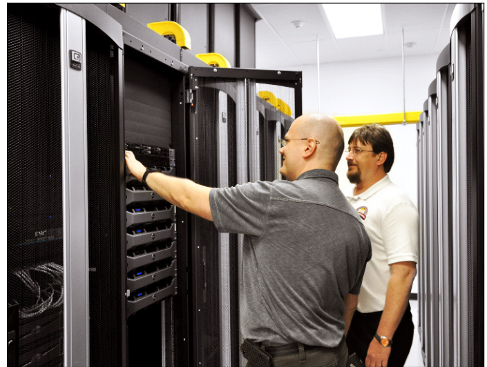
Robert Carneim, PhD, Supervisor of Instructional Technology and Doug Cofer, Data Center Director for Oak Ridge Schools chose CPI F-Series TeraFrame® Cabinets with Vertical Exhaust Ducts and custom grommets to keep the room temperature in their data center effectively cool.
