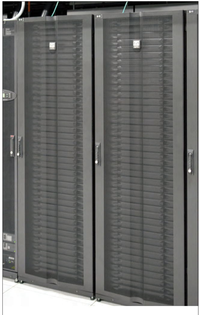
CPI's GF-Series GlobalFrame Cabinets with custom doors, support baffles and Hotlok® Snap-In Filler Panels were installed to improve airflow efficiency in Cologix's Dallas data center.
