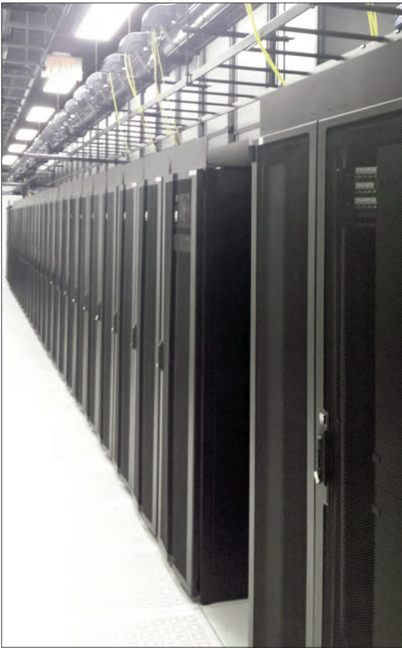
CPI's GF-Series GlobalFrame Cabinets with Vertical Exhaust Ducts were a part of the total Cologix solution (Vancouver site).
