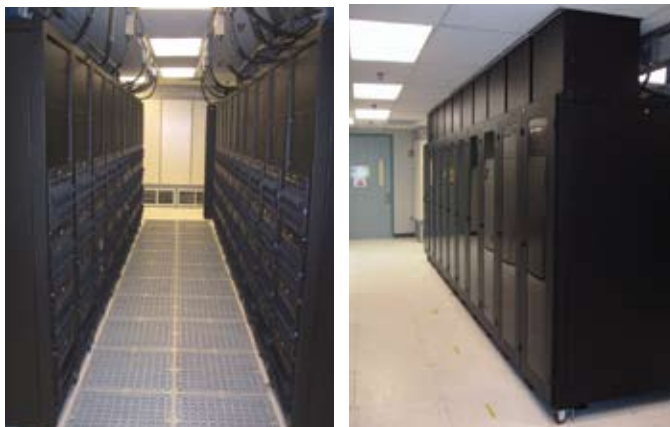
Figure 6 (hot) and 7 (cold). The basic cabinet can dissipate even more heat under appropriate circumstances.
