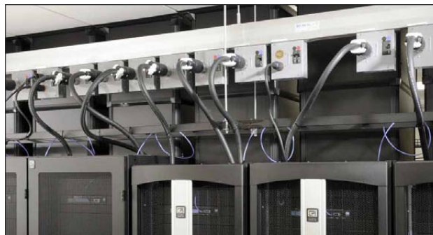
StarLine Overhead Electrical Distribution
