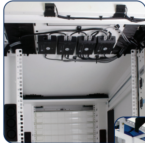
Above: eConnect Sensor Array installed in a CPI ZetaFrame® Cabinet System.
