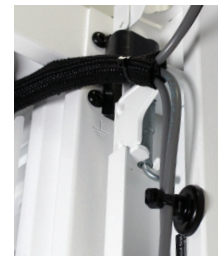
Sensor Installed in ZetaFrame Cabinet
