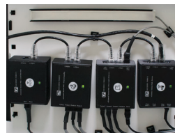
Cabinet Work Light and Sensors installed in Cabinet
