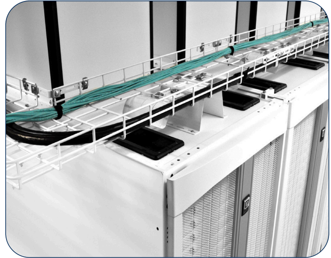
CPI's Wire Mesh Cable Tray provides point-to-point pathways for the network cabling in the data center.
