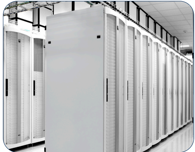
CPI's F-Series TeraFrame Gen 2 and N-Series Network Cabinets in Glacier White brighten UF Health Shands' data center and provide better visibility, while reducing power costs.
