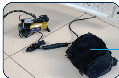
6 ZutaCore HyperCool Support Kit: Utility service unit used to pressure-test the system.
