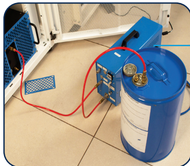
4 ZutaCore HyperCool Service Unit: Utility service unit used to pump liquid coolant into the HRU and to purge non-condensable gases out of the system.
