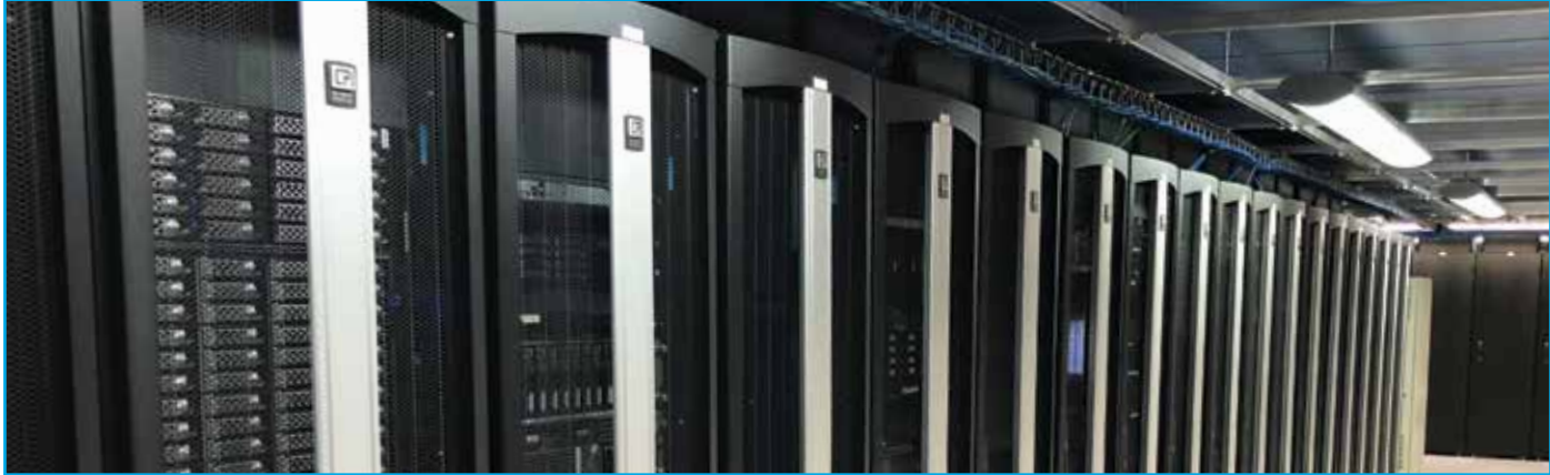
F-Series TeraFrame Cabinets with Vertical Exhaust Ducts are the standardized solution in Xfernet’s Los Angeles data center.
