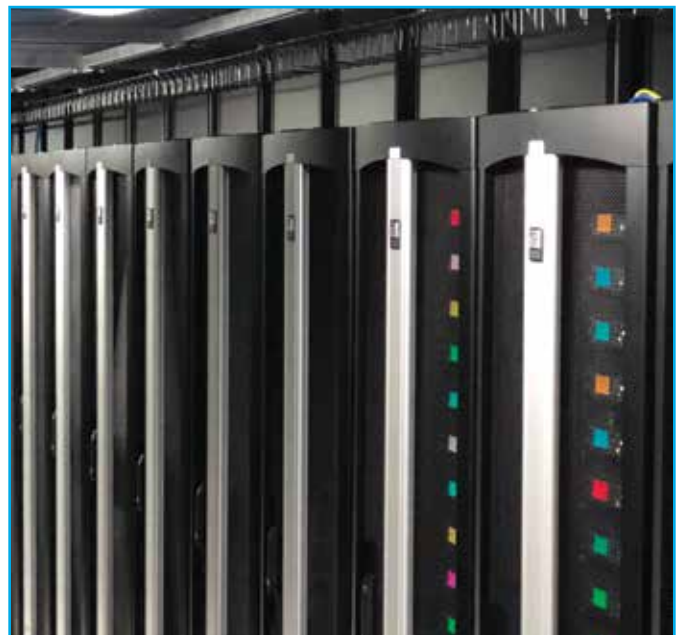
Increasing demand for higher rack densities drove Xfernet to deploy a reliable data center infrastructure comprised of cabinets and cabinet-level containment.
