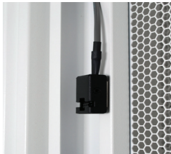
Sensor Installed in ZetaFrame Cabinet
