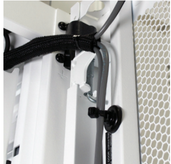
Sensor Installed in ZetaFrame Cabinet.
