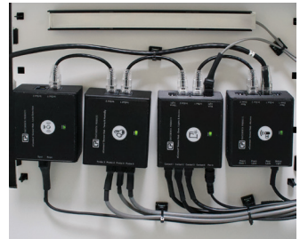
Cabinet Work Light and Sensors installed.
